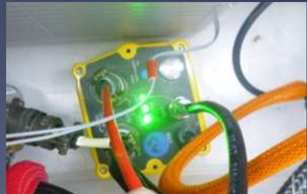
XI-202 installed at ICE-Z site on Mt. Erabus
