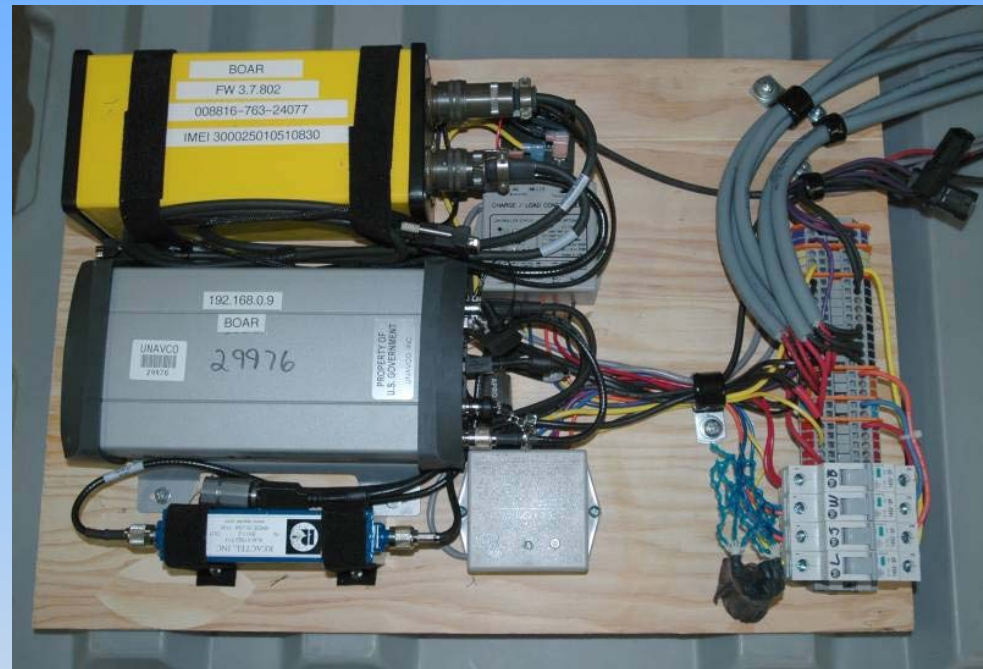
XI-100 on GPS electronics board installed at Pine Island Glacier station BOAR
